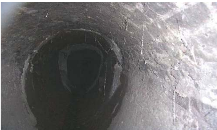
Water can "infiltrate" water pipes through leaks in pipe joints and connections or through breaks and cracks.
